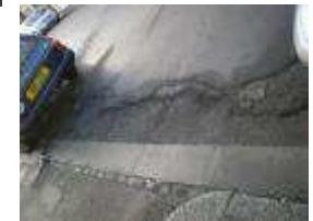
Poor state of carriageway on Lugard Rd.
